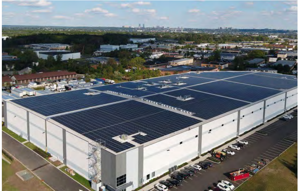
Community solar puts panels on warehouses, not homes, bringing energy and other benefits like cost savings to residents. The solar panels on this warehouse owned by Prologis, that recently acquired prior building owner Duke Realty in Wood-Ridge are now powering Jersey City homes.
